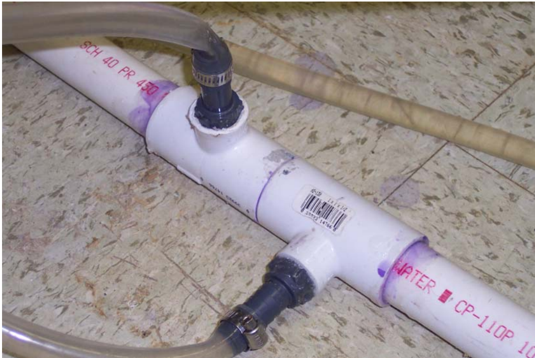
Figure 3. Monitoring and water use node
