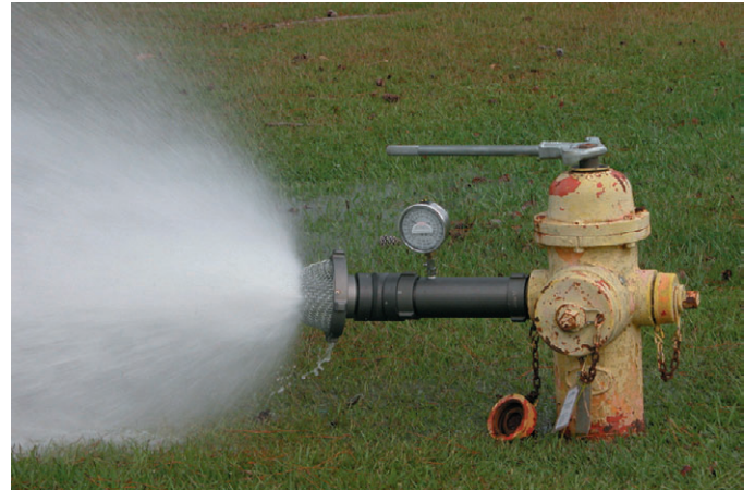
Figure 4-6. A Hydrant Being Flowed with a Diffuser as Part of a Fire-Flow Test.
